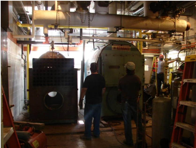
Photos: Contractors from LBP Mechanical of Minneapolis work on Pine Technical College's boilers.
